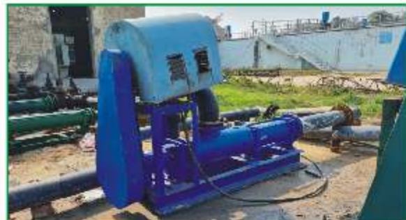
ETP- Sludge Transfer-UAE
